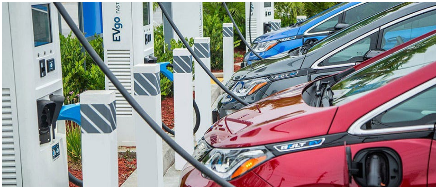
An electric vehicle charge station.
