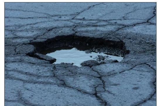
Figure 1. AC Stripping Damage in Flexible Pavement in Louisiana
