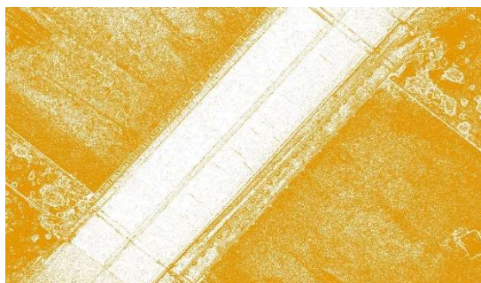
Figure 2. Cracking Highlighting Image
