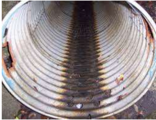
Figure 1: A corroded metal culvert
