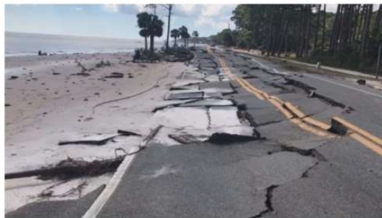
Figure 1: Extreme damages to pavement built using cohesionless soils near the coastal region of southern United States
