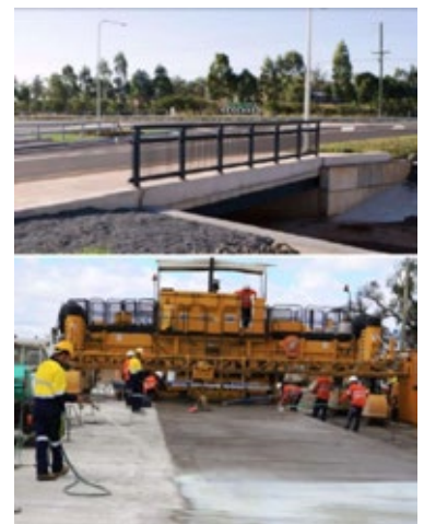
Bridge and pavement construction using GPC concrete at Brisbane West Camp Airport, Australia.
