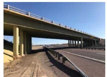
Bridge in Socorro, New Mexico, where the UHPC overlay will be implemented.
