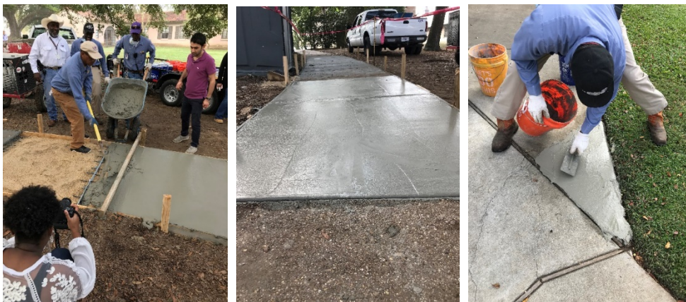
Figure 1: ECC Field Study (a) ECC Sidewalk Construction (b) Finalized ECC Sidewalk (c) Repair of Cracked Sidewalk Using ECC.
