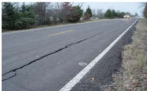
Figure 1. Paris, TX site longitudinal shrinkage cracks.
