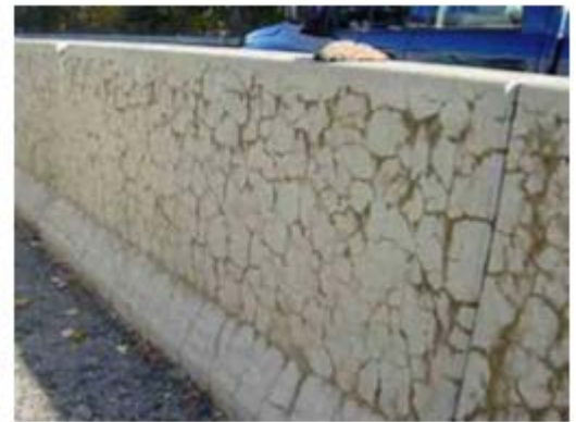
Figure 1. Concrete structure damaged by sulfate attack.
