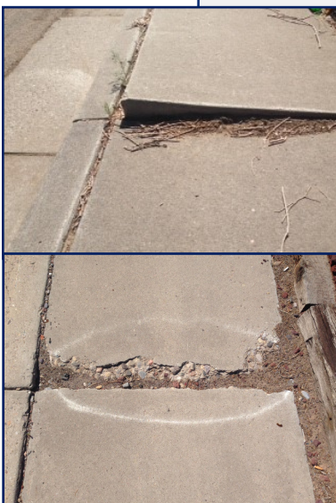
Typical sidewalk defects in Albuquerque, NM
