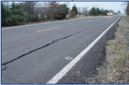
Paris, TX site with longitudinal shrinkage cracks
